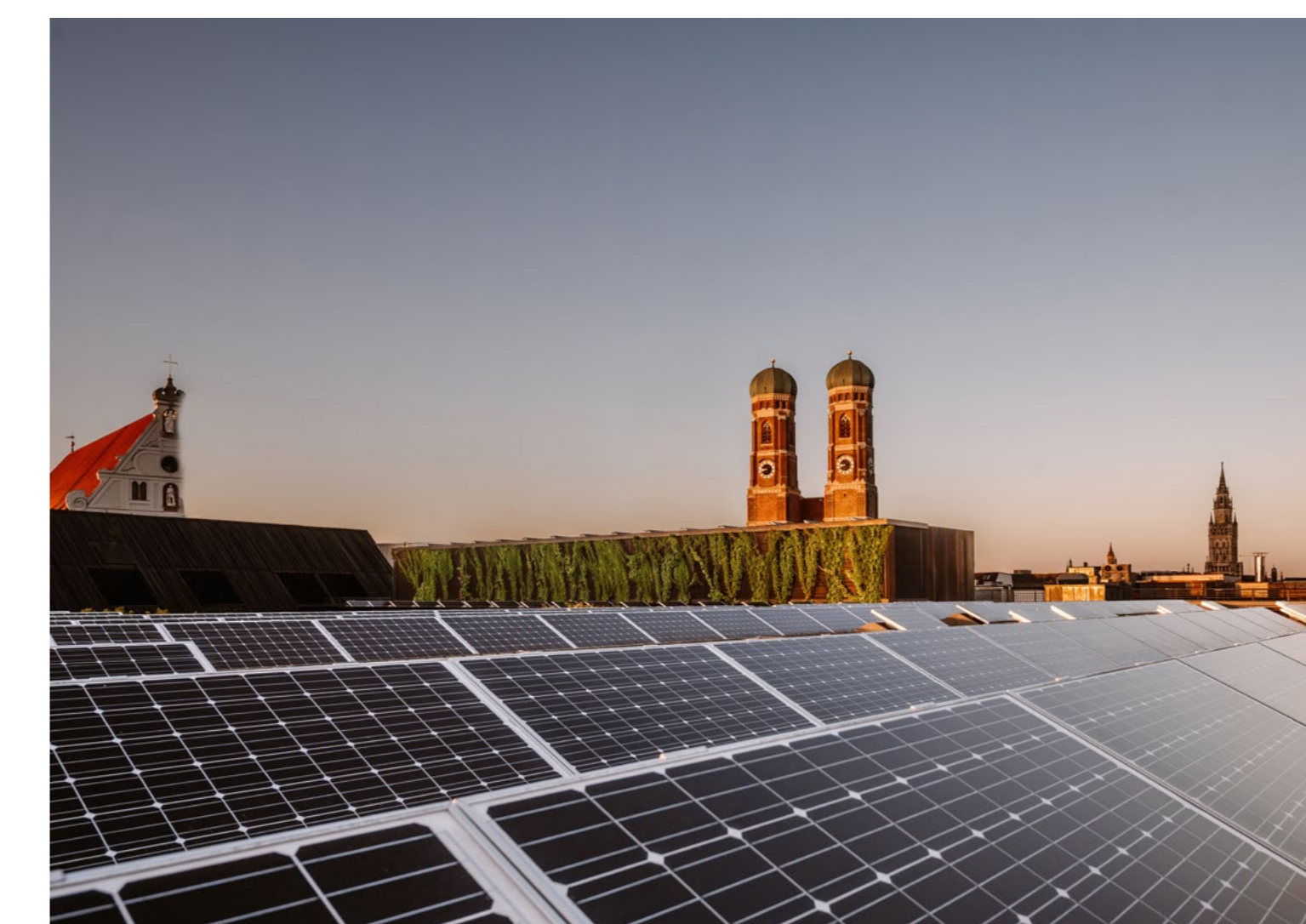
Photovoltaik Joseph Pschorr Haus
